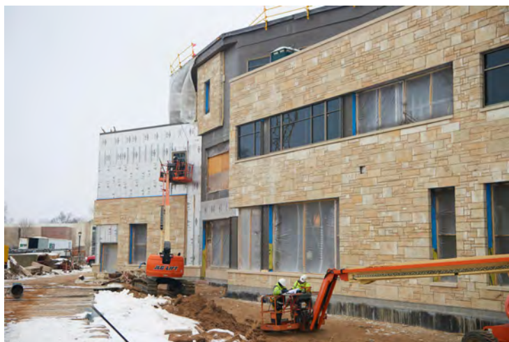
Contractors work on the south entrance of the student center. The edifice is designed to emulate Grandad Bluff.
