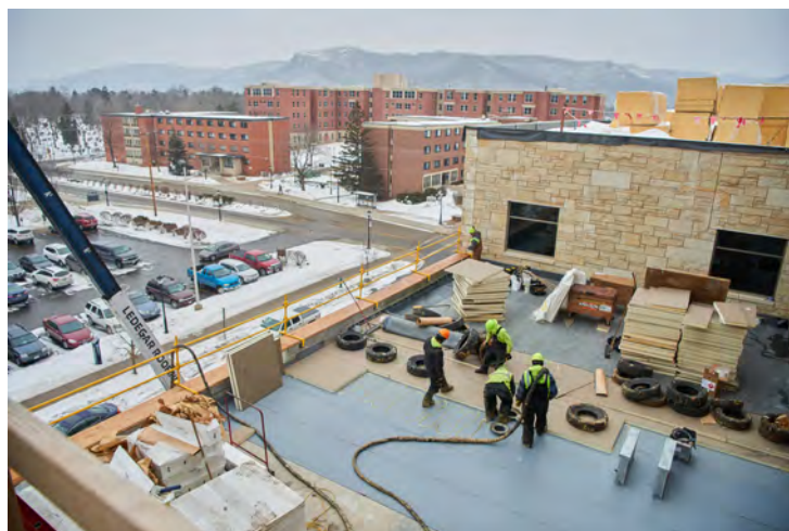
Workers place insulation on the roof of the student center. The building will incorporate a sustainable design strategy with the goal of achieving Leadership in Energy and Environmental Design (LEED) Gold Certification.
