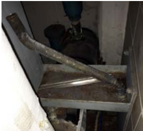
④ Chilled water entrance near floor in bakery
