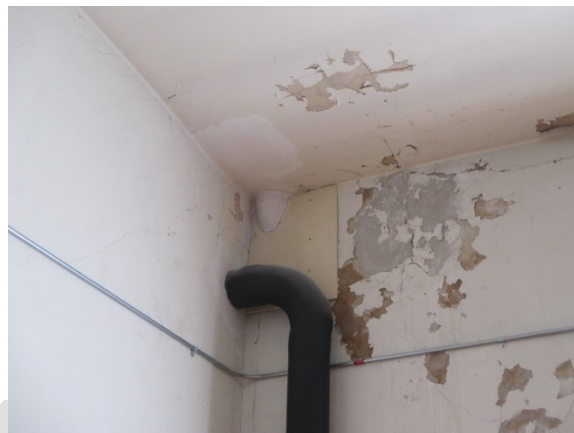
Water Damage at Gymnasium Ceiling – 1916 Wing (2014)
